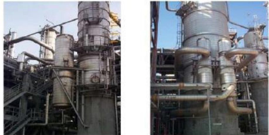
Vertical Thermosiphon (UOP)
