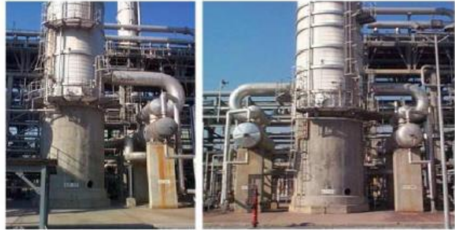
Horizontal Thermosiphon (UOP)
